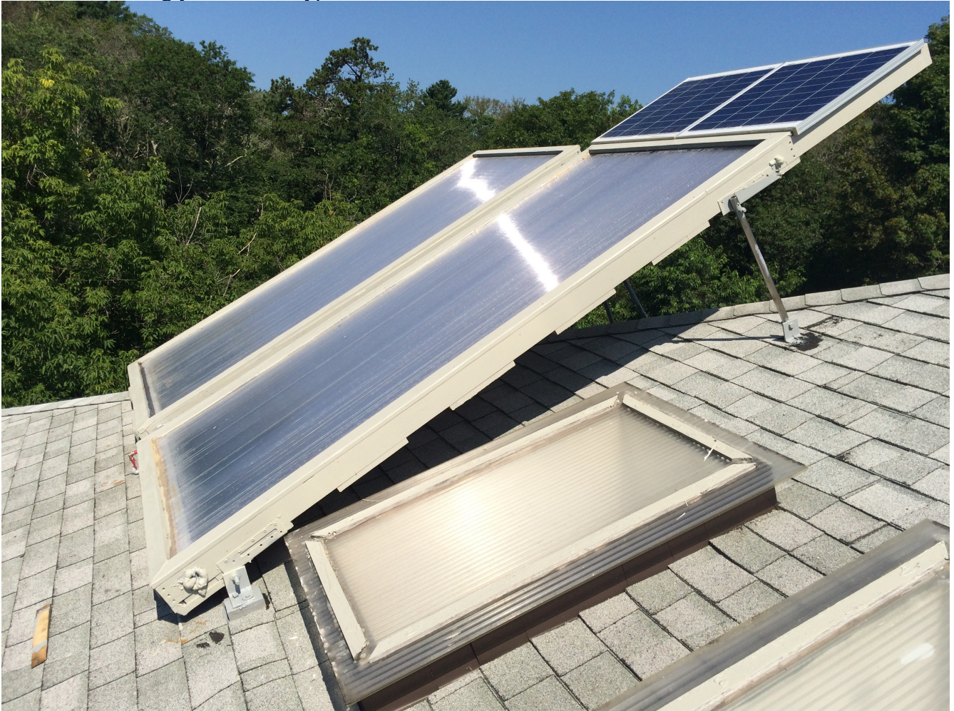
Here is a view of the collectors looking west
